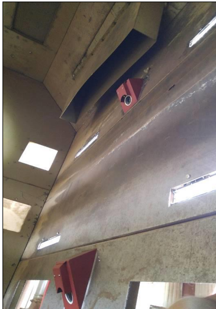
Figure 1. Photo of USDA ARS Module Feeder Inspection System IP cameras installed in back wall of module feeder dispersing cabinet at Gin A.
